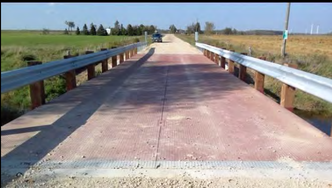
Photo 7: Galvanized expansion joint interface with cover and bridge deck of 18.3m span Lessard Modular bridge.
