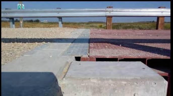
Photo 8: Close-up of galvanized expansion joint interface with protection plate on the road side of the ballast wall. Not visible - Dow Corning 902 RCS over the 50 x 50 Eva foam joint.
