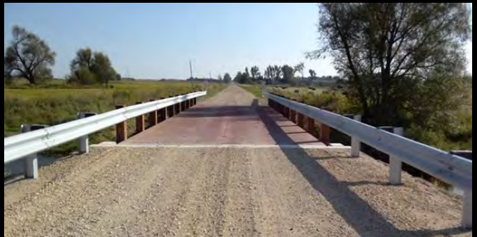
Photo 6: North approach to new 18.3m span Lessard Modular bridge with custom expansion joint with new flex-beam.
