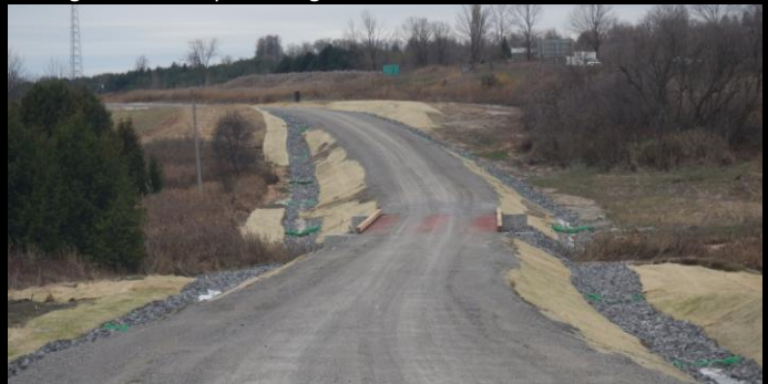
Photo 4: View looking west of new 15.2m span x 6.1m wide Lessard Modular bridge with completed abutments and wing walls.
