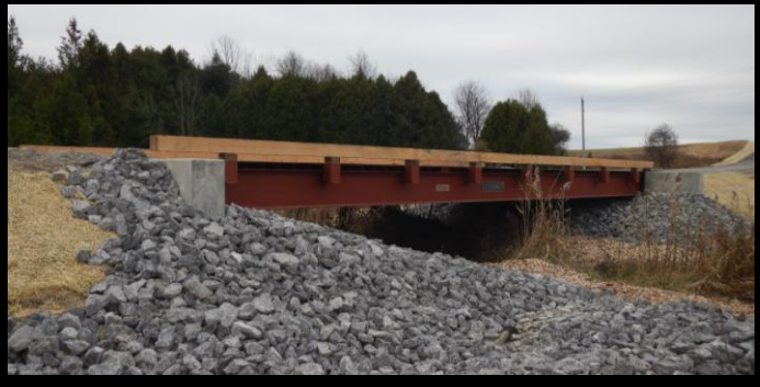
Photo 6: Upstream face of new 15.2m span x 6.1m wide Lessard Modular bridge.
