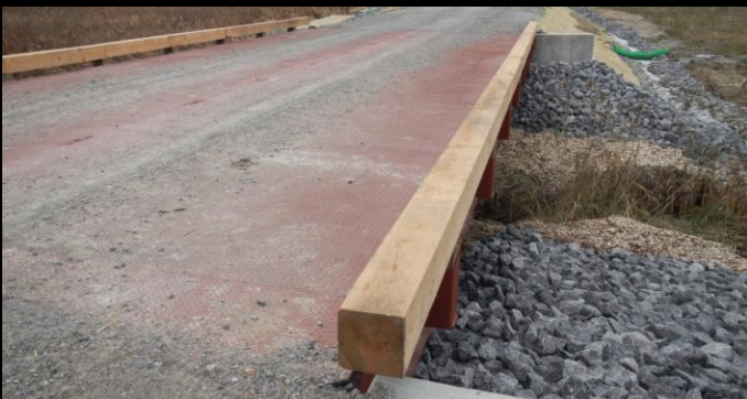
Photo 7: Close-up view of the North east corner of the new 15.2m span x 6.1m wide Lessard Modular bridge.
