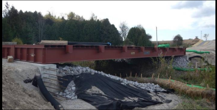
Photo 2: Upstream face of new 15.2m span x 6.1m wide Lessard Modular bridge. Westerly view of newly installed modular bridge on new concrete bearing - with incomplete wing walls.
