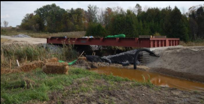
Photo 3: Upstream face of new 15.2m span x 6.1m wide Lessard Modular bridge. Easterly view of newly installed modular bridge on new concrete bearing - with incomplete wing walls.
