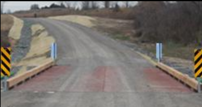
Photo 5: Close-up view looking west of new 15.2m span x 6.1m wide Lessard Modular bridge with completed abutments and wing walls.
