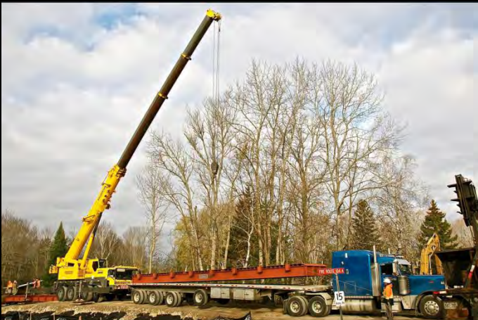
Photo 7: 90 Ton Crane lifting section 2 of 2 of new 15.2m Lessard Modular bridge off of tractor trailer for placement on bridge.
