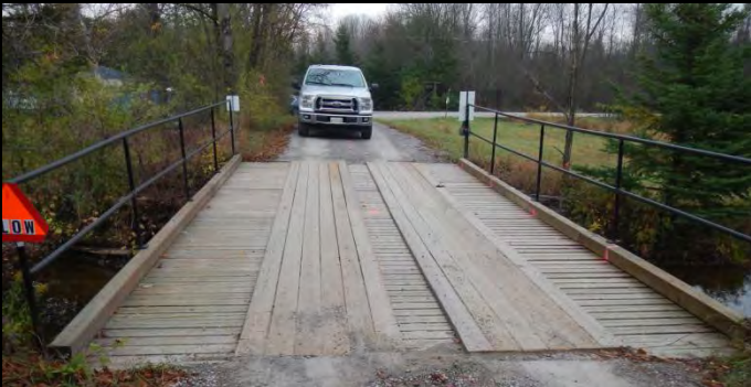
Photo 5: West approach to existing bridge with handrail and no Wa33 Signs.
