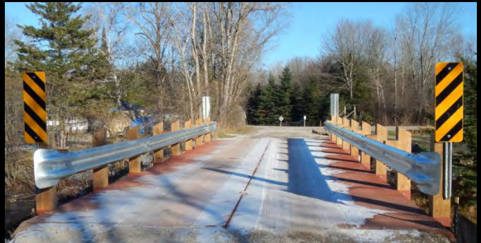
Photo 6: West approach to new 15.2m span Lessard Modular bridge with Wa33L/R signs and flex beam rail.
